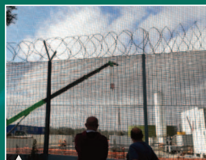
Two environmental HRDs from the NO TAP movement visit the TAP building site in Puglia (Southern Italy).
